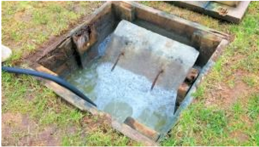
Figure 7.1 Tank adjoining tile drainage system where the resonant sensor could be potentially deployed
